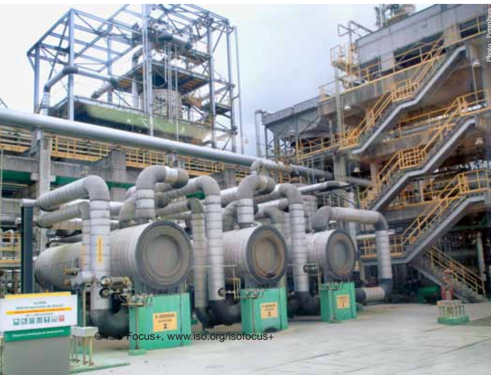
Petrobras' diesel hydrotreating unit.
