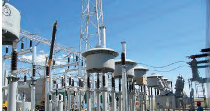
Figure 4-6 – 750 kV CSR at the Dunhuang substation, NW China (SGCC)
