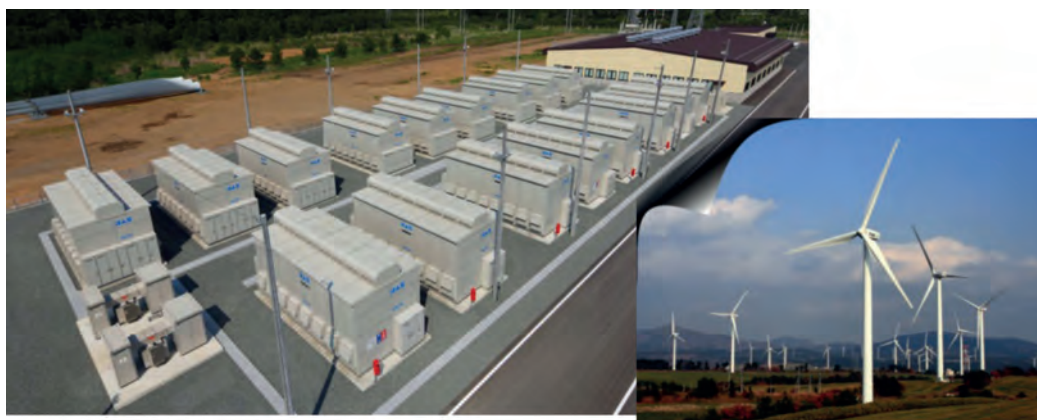
Figure 5-7 – JWD’s wind and NAS battery hybrid system in Japan (NGK)
